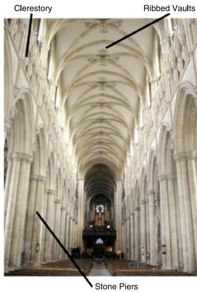
Fig. 1. The interior view of the nave of the Beverley Minster displays the limestone piers that support the stone vaulting. The leaning of the columns outwards is visually observable on site.
